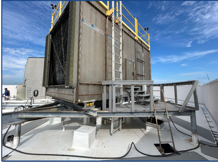
Photograph No. 15: Elevated main AC unit located at the center of the roof.
