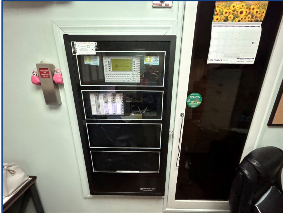
Photograph No. 26: Fire alarm control panel located in the office area.
