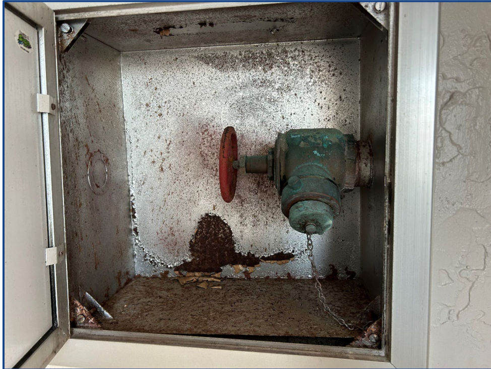
Photograph No. 20: Typical standpipe at hallway for water access.
