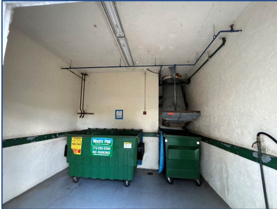
Photograph No. 24: Typical trash chute room.
