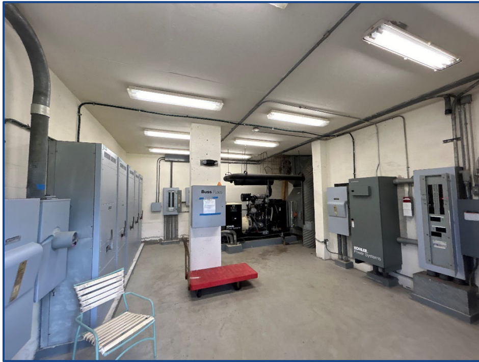
Photograph No. 25: First floor utility room at the south side of the building.
