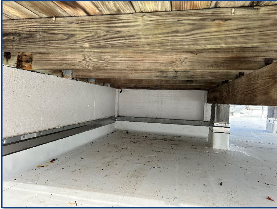
Photograph No. 17: Wood roof deck at the west side of the roof with rusted clips and bolts.
