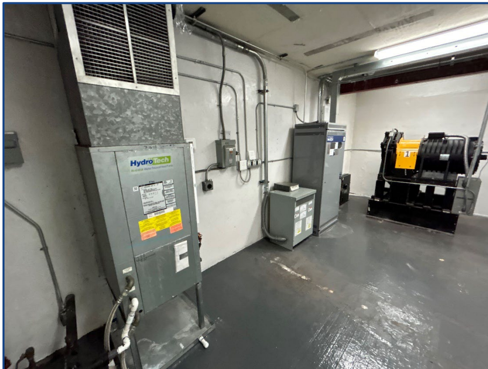
Photograph No. 22: Overall roof utility room with elevator panels and units.
