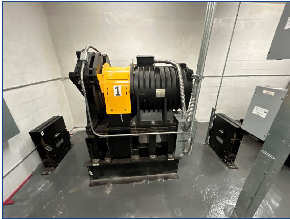
Photograph No. 23: Elevator traction machine located at the roof utility room.
