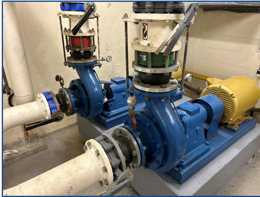
Photograph No. 21: Motors located at the roof.
