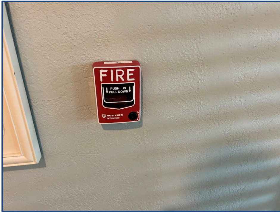
Photograph No. 19: Typical fire alarm located in the lobby.
